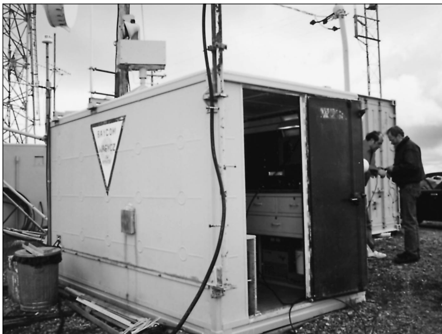
The W6WX/B housing on Mt Umunum. K6GSJ (l) and N6EK (r) are working on some of the coaxial cabling. The GPS unit is mounted on the pole at the far left corner of the housing.
